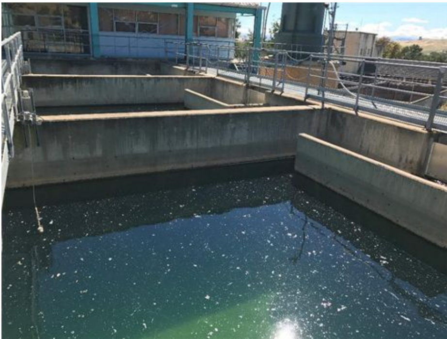
Figure 13-4 Jugiong Water Treatment Plant - Filters
