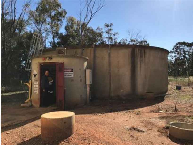
Figure 15-4 Mt Arthur – Chlorination and Ganmain low level reservoir
