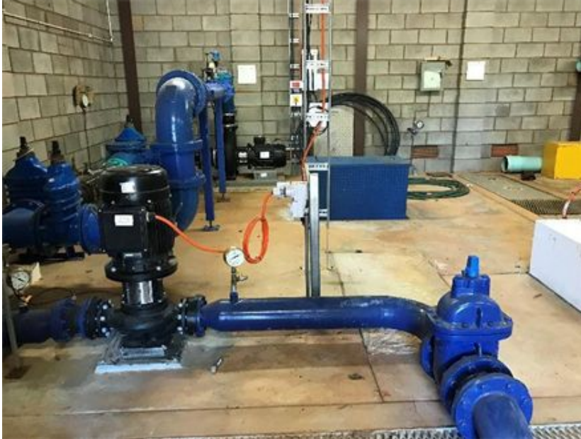
Figure 15-6 Mt Arthur – Ganmain pump station
